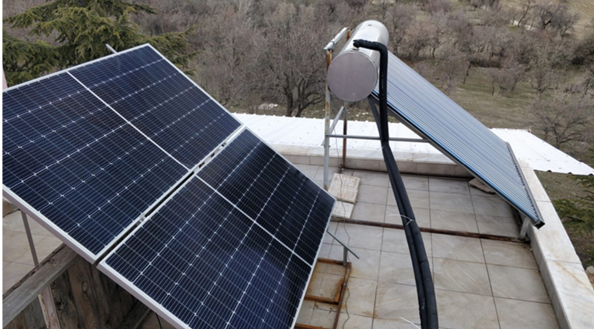
Figure 4. PV panels and vacuum solar collector used in the experimental setup
