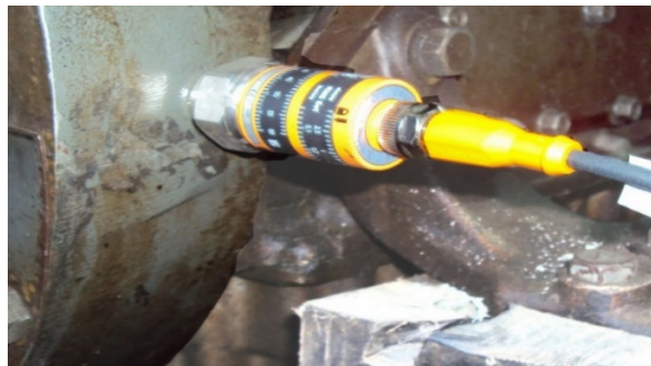
Fig. 6. Location of vibration sensor installation
